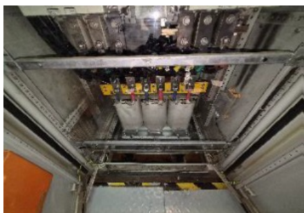
Bow thruster control cabinet
