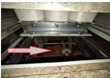
Cooling pipeline located directly below the cabinet
