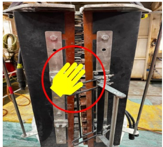
Showing the pinch point on the Induction Heating Coil
