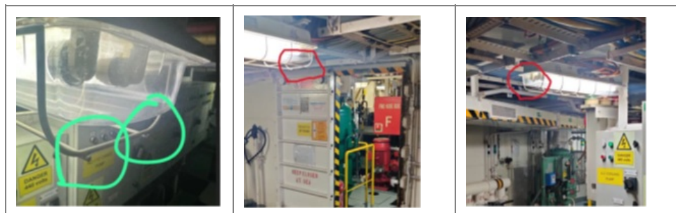
Location of lighting and lighting protection grille rod hazards.
