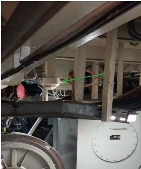
Smoke detector over the affected Shaft Generator
