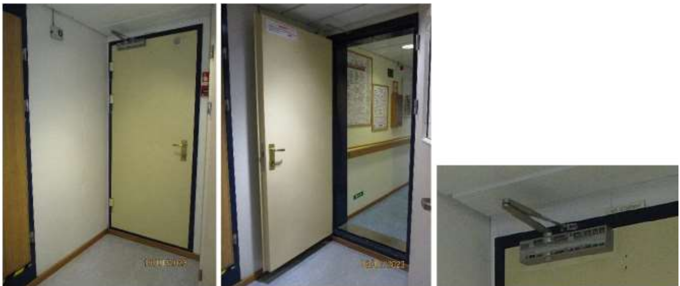
Fire Doors and Closing Mechanism
