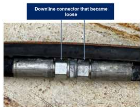
BSP fitting which came loose
