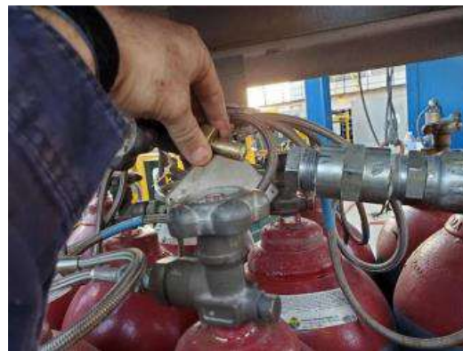
Incident 2: Failed Hose Connection on Bottle Rack.
